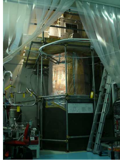
Figure A.30: The LArGe setup with fully installed cryogenic system, lock, and a scaffold with a working platform.
