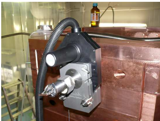
Figure A.23: Orbital welding of the cryo-tubes on site, after one part has been pushed through the shielding.
