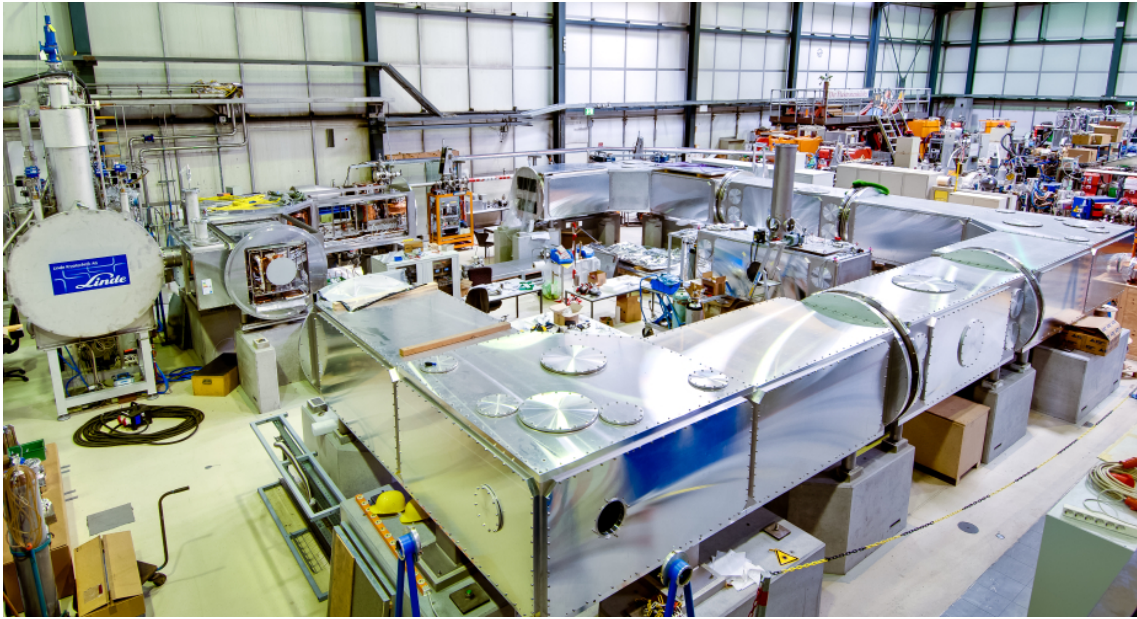
Figure 5.2: Photo of the CSR construction site (as seen from the left side of Fig. 5.1): The helium refrigeration system on the left side is connected to the first finalized corner for cryogenic tests. Most isolation vacuum chambers are in place, and the inner vacuum chambers of these sections are presently being installed.
