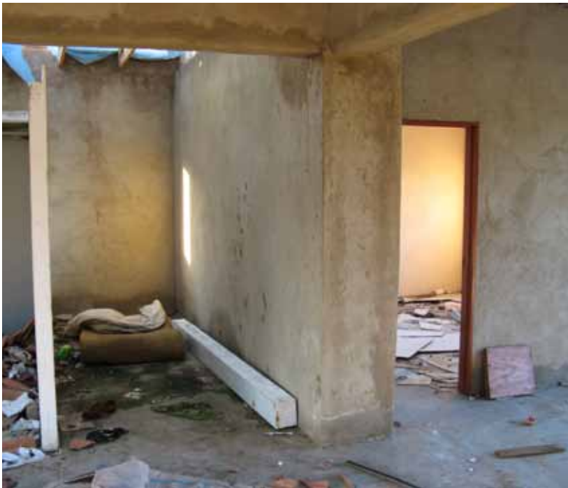
Photo 13: The vandalised cold room
