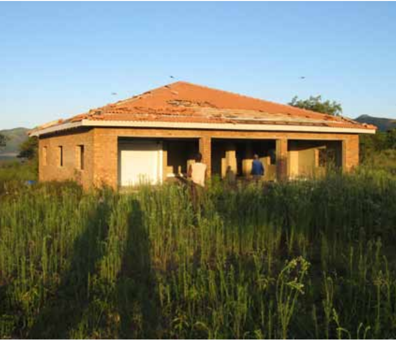
Photo 10: Vandalised office building
