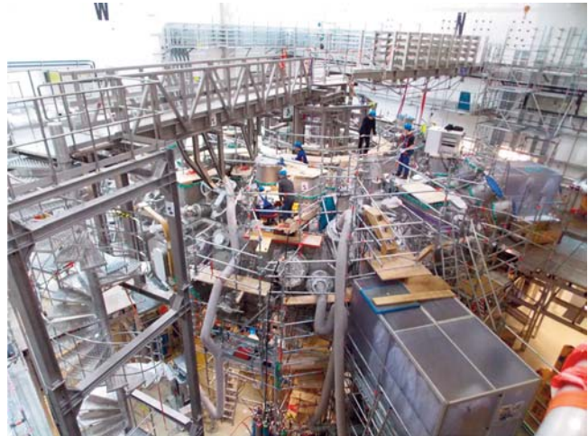
Figure 12: Wendelstein 7-X with periphery and first diagnostics (auxiliary structures, cable trays, pipe-systems).
