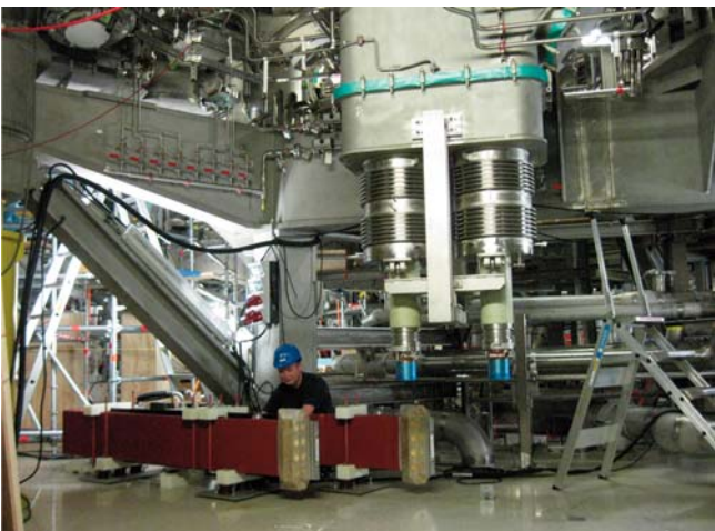
Figure 9: One CL-pair, protruding out of the CL-dome with bellows and pivot-bearings; below: aluminium bus-bars during the installation.
