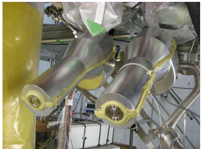
Figure 15: Test chambers at bus-bar joints.
