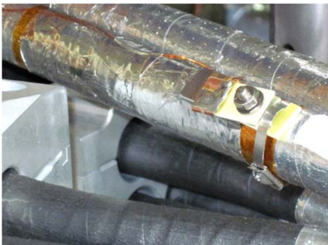
Figure 13: Collision sensor placed between a bus conductor and a support clamp.
