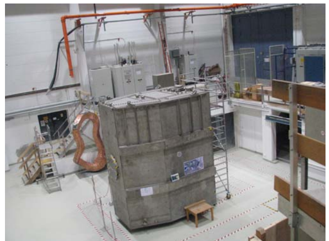
Figure 1: View into the refurbished old W7-AS experimental hall with the first installation work for ELISE (target tank). The outer red lines on the floor indicate the position and the area of the concrete neutron shield.
