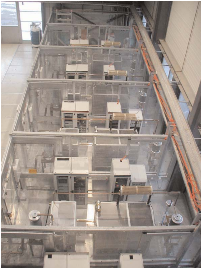
Figure 36: High Voltage Installation in the ECRH-hall at IPP Greifswald
