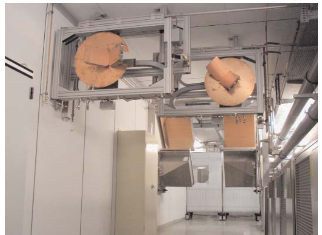
Figure 37: The retro-reflectors in the beam duct at IPP, a set of MBWG-mirrors and microwave absorber panels are seen in the background
