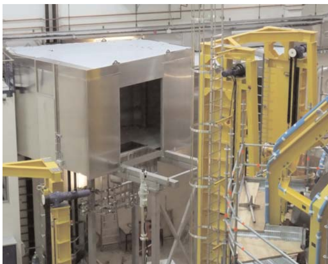
Figure 31: High voltage cabin for NI20 installed on its support structure inside the torus hall, the second cabin for NI21 is hidden behind the port installation tower.
