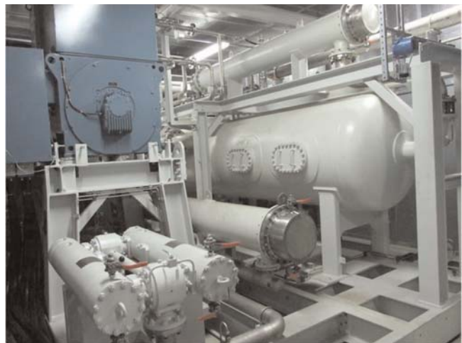
Figure 5: Electrical drive with oil separator, oil cooler and filter of the screw compressor unit.
