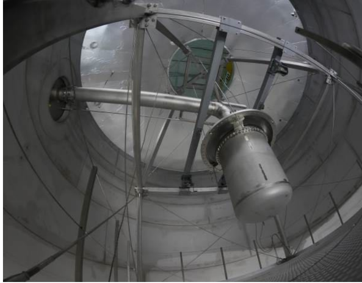
Figure 2.8: The picture shows the cryostat as it is mounted to the transport pipe. The top of the outer vessel is already installed but the vessel itself will be assembled later. The entire system of cryostat and pipes is installed inside the water tank.
