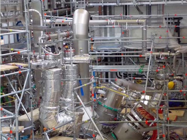
Figure 8: One double vacuum pump-unit out of five at the upper side of the machine; the chimney to the right is the redundancy to the safety-valves that protect the cryostat from over-pressure.
