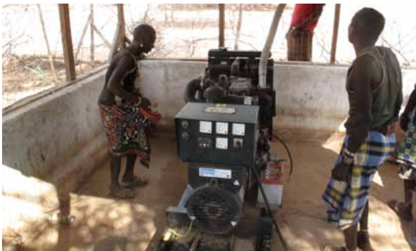
Photo 3: The water pump for which Isir has procured the battery.
