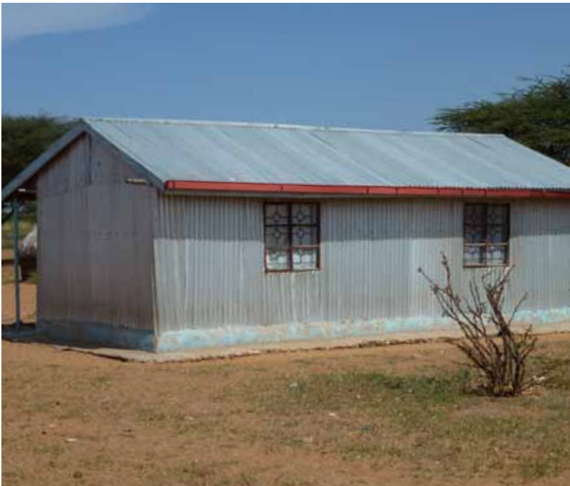
Photo 7: This house belongs to an NGO worker. It is built entirely of corrugated iron sheets nailed to a wooden frame. (I. SCHLEE, 20140611Korr, P1010538, P1010539.JPG)
