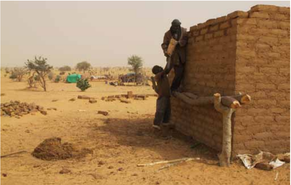
Photo 158: Building a mud brick house in a rural Wodaaße centre . Salaga, Damergou region. (F. KÖHLER, 2011)
