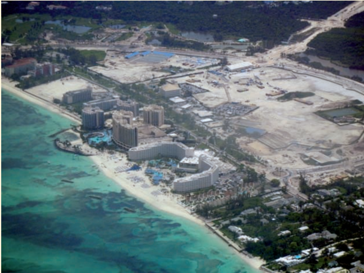
Fig. 18: New beach resort ('Baha Mar') development at Cable Beach, Nassau (Photo: A. Holdschlag 2011)
