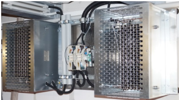
Fig. 6: Discharge unit (2 dump resistors and DC power contactor with normally closed main contacts)
