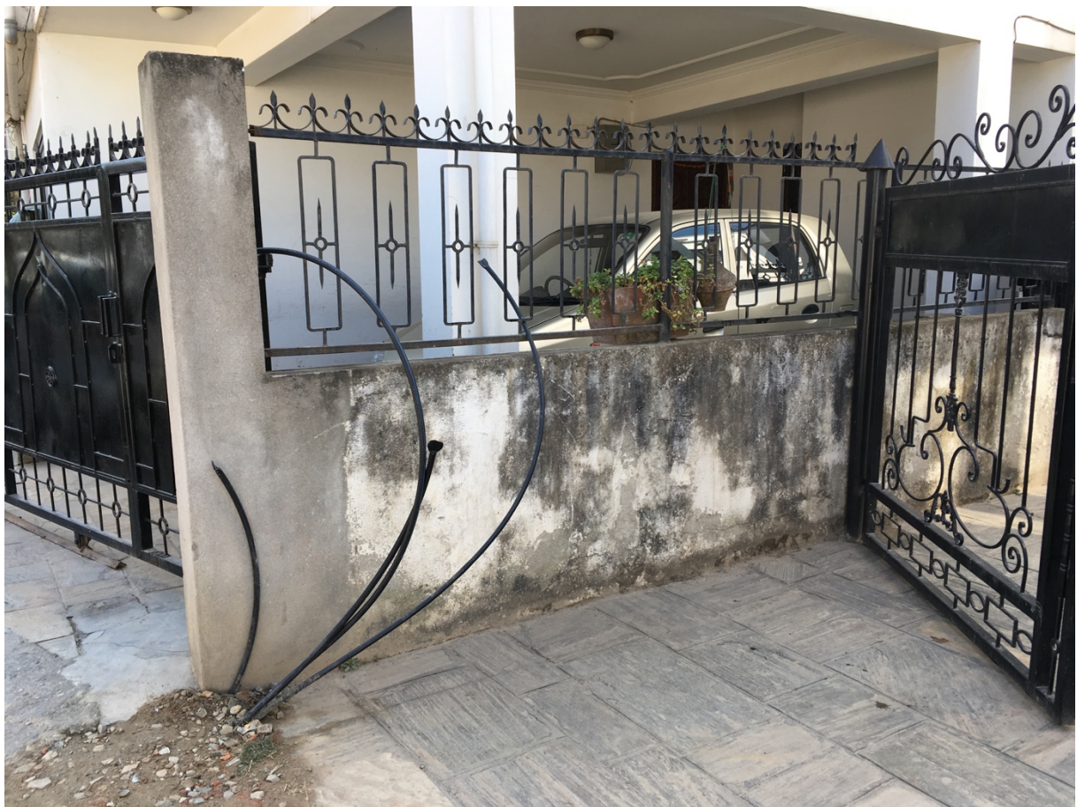
Figure 2: The PVC pipes waiting for Melamchi's water, 29 February 2017, Sanepa, Kathmandu Valley.
