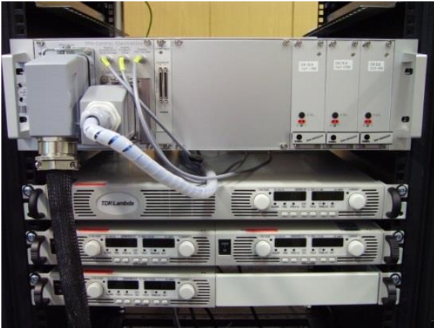
Fig. 8: Photograph of the electronics system providing operation of one DPG head.
