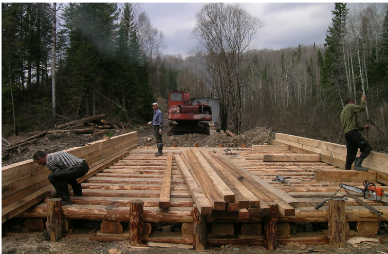
Fig. 2.7. Bridge-building for a new road in the Saian Mountains (Kuraginskii Raion). Photograph by Dennis Zuev, 6 May 2009, CC-BY.
