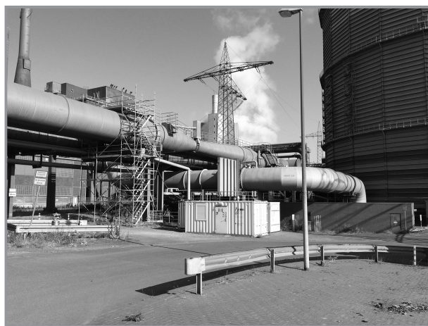
Figure 6. HüGaProp containers at the steel mill plant of thyssenkrupp Steel Europe in Duisburg.
