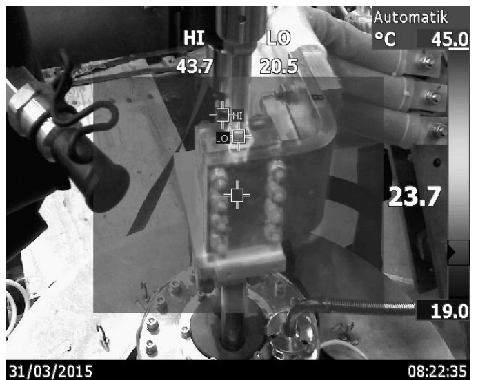
Fig. 6 Thermal picture of the connection area during heat run. The hot spot (HI) with 43.7 °C is inside the clamped copper block where the contact lamellas are located.
