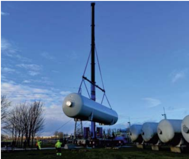
Figure 11: Transportation of the new helium gas storage tank to the final place close to the other four tanks.
