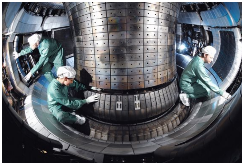
Figure 2.1 – Interior view of the ASDEX Upgrade tokamak during installation of the tungsten plasma facing components (source: IPP web-page).
