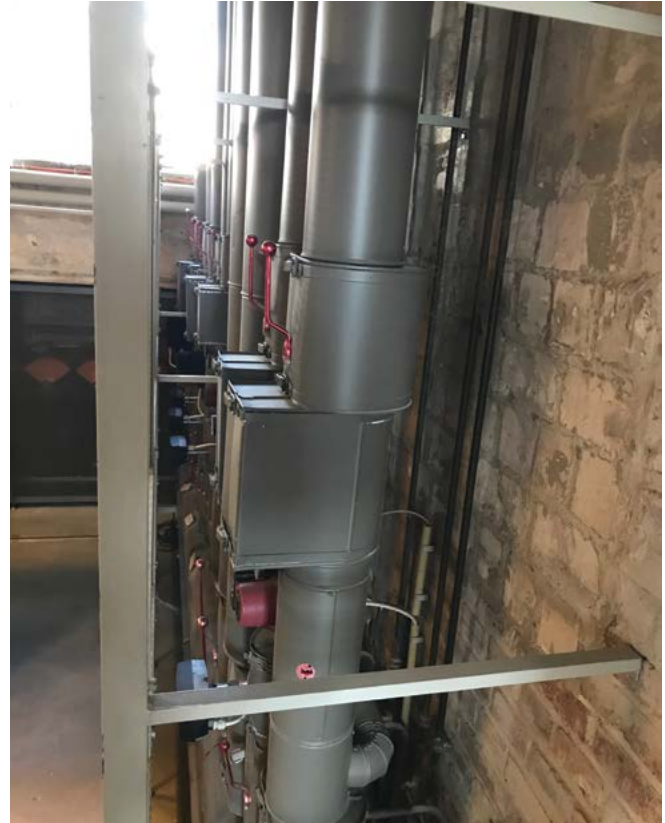
FIGURE 6: A PHOTOGRAPH OF THE DISTRICT HEATING CONTROL AND MAINTENANCE ELEMENTS, BAUHAUS DESSAU, 2019
