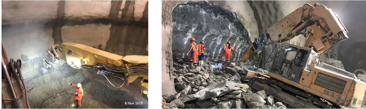
Figure 10.54: Left: Roadheader being used for shaft excavation at HL-LHC Point 1. Right: Rockbreaker used for new service tunnels excavation at HL-LHC Point 5 (Credit: Z. Arenas).
