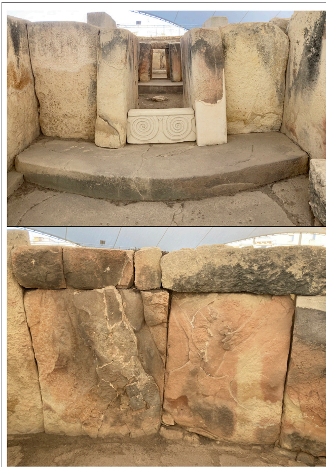
FIGURE 6 | Tarxien temple. Note fire damage (reddened areas).
