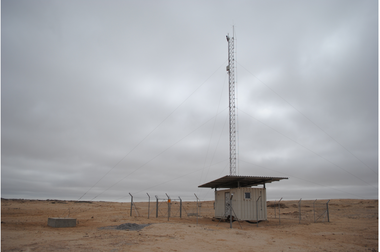
Figure 27: Air measurement and sampling station at Gobabeb, Namibia.
