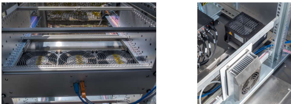
Figure 53 Left: Customised fan tray in a 2U housing. Right: Dehumidifier (silver housing) with a small hose for the condensate. 400 W fan heater (black housing) installed at the floor of the cabinet.
