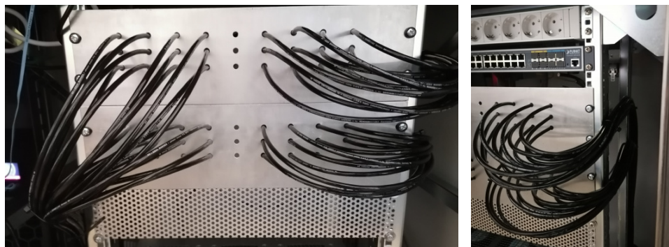
Figure 49 Left: Front view of the cable routing inside a cabinet with 19-inch rack. On the left half the cables are fed from below and on the right half from the back. Right: Photo of the cables fed in a single bundle from the back of the rack to each half of the PhantomHV dummies.
