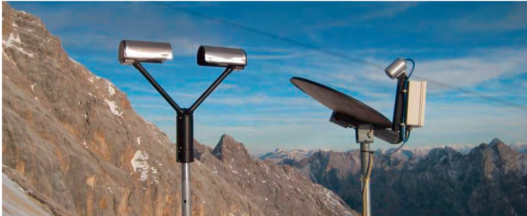
Fig. 3: Installation of the PARSIVEL-2 disdrometer (left) and MRR micro rain radar (right) at the top terrace of the Umweltforschungsstation Schneefernerhaus. Photo by M. Hagen.
