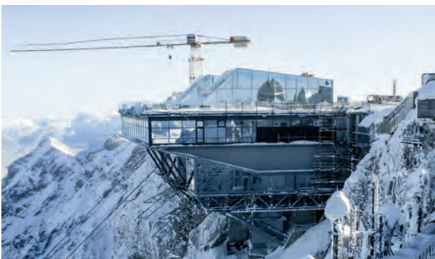
Fig. 19: Construction site of the new summit station for BZB’s “Seilbahn Zugspitze” (“Cable Car Zugspitze”)
