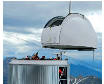
Fig. 26: Installation of the large laser tower for the RAMAN-LIDAR on the roof platform of the UFS building (2010)
