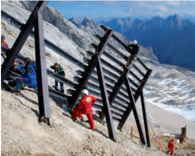
Fig. 23: View of the construction site for the integrated rockfall and avalanche protection system for the high-altitude research station UFS (see also Fig. 25)
