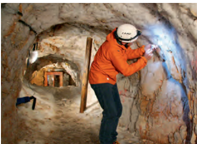
Fig. 24: Permafrost measuring system, installed in the remaining summit tunnel between the UFS and the former terminus of the "Austrian Zugspitze Cable Car"
