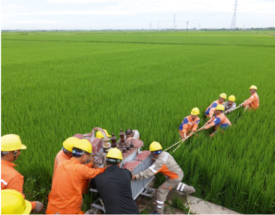
Vietnam Electricity workers remove an old transformer to make way for one of higher capacity. (Photo: Thi Phuong Thao Vu, 2019)
