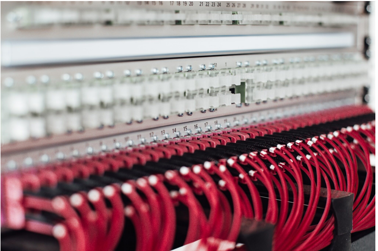
Fibre optic cable rack . Photo by Lars Kienle, free to use under the Unsplash License.
