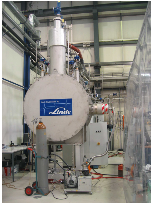
Figure 3.12: The connection box of the refrigeration system is shown and the cold box is located behind. The red and white striped area on the right is the position where the CTF was connected later.
