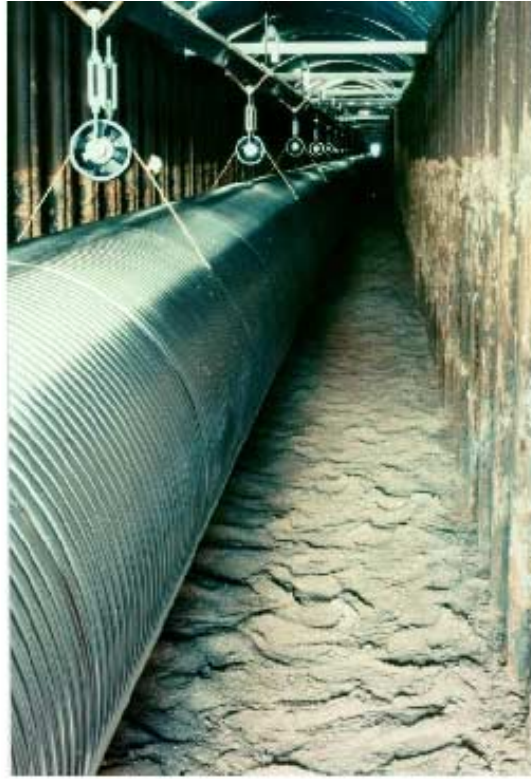
Fig. 4. The convoluted tubes during installation; with each new 4.5 m piece welded on, the tube was slid 4.5 m further into the 600 m long trench, using trolleys along the aluminum rail at the top.
