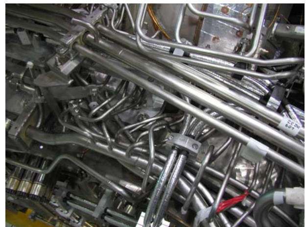
Fig.4 Impression about the assembly conditions of the cryo pipes
