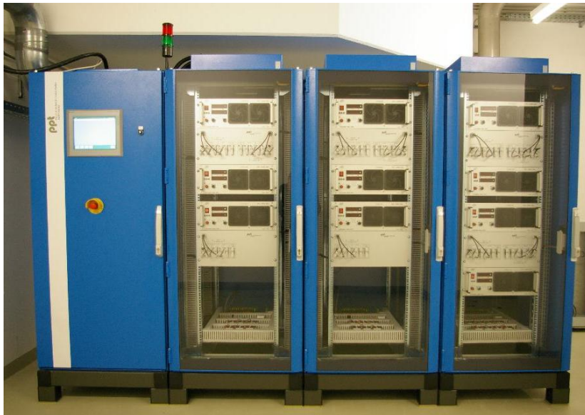
Fig.2 Power supply system after installation.
