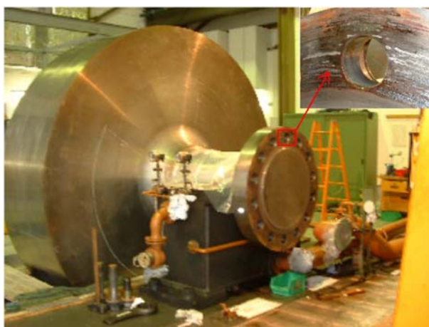
Fig. 2 Damage at coupling of EZ4
