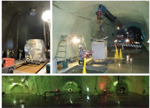
FIG. 2. Some photos in the KAGRA facility. Top Left : installation of cryostat underneath the vertical borehole for the 2-story suspension tower. Top Right : installation of the granite stone for the geophysics interferometer. Bottom : panorama of the KAGRA tunnels from the central station right after paving the floor.
