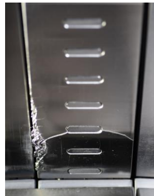
Fig. 9. Picture of a broken tile embedding Langmuir probes in AUG with strongly damaged leading edge (sector 8).
